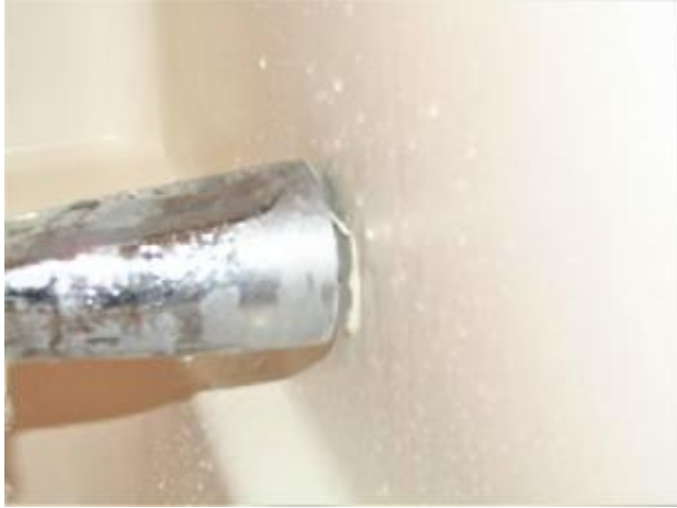
The showers in both of the upstairs bathrooms do not work properly and the faucets need sealed to the wall.
