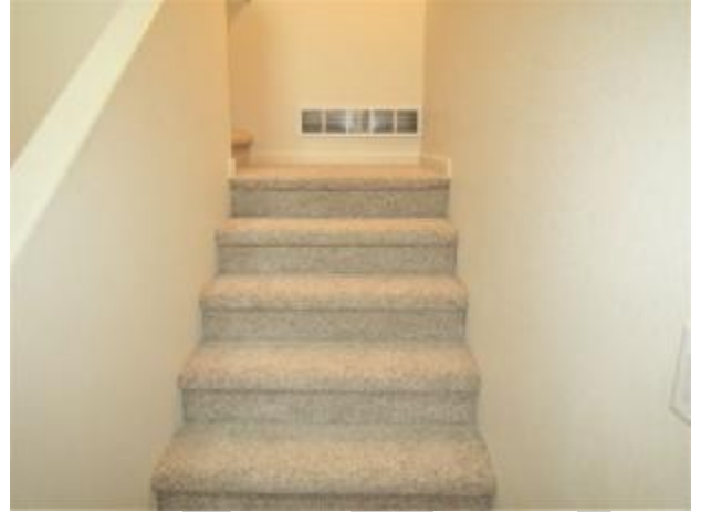
A handrail for the lower set of steps needs to be installed for safety.
