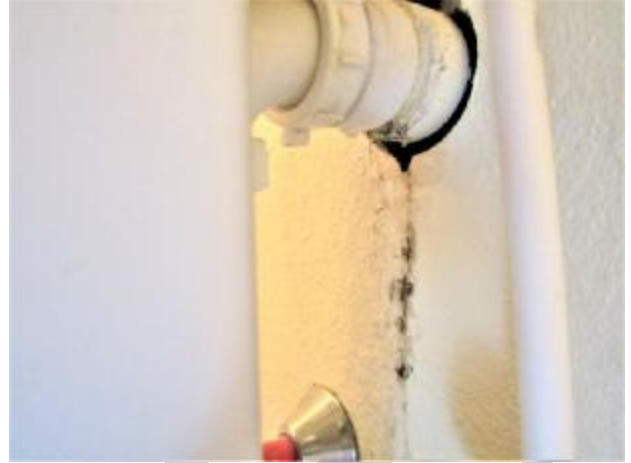
The sink in the downstairs bathroom is loose from the wall and the floor. The sink drain is leaking.
