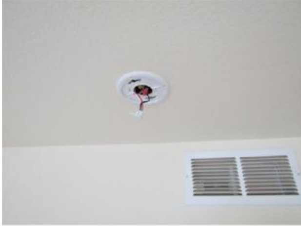
The smoke detector is missing in the master bedroom. Install smoke detector for safety.
