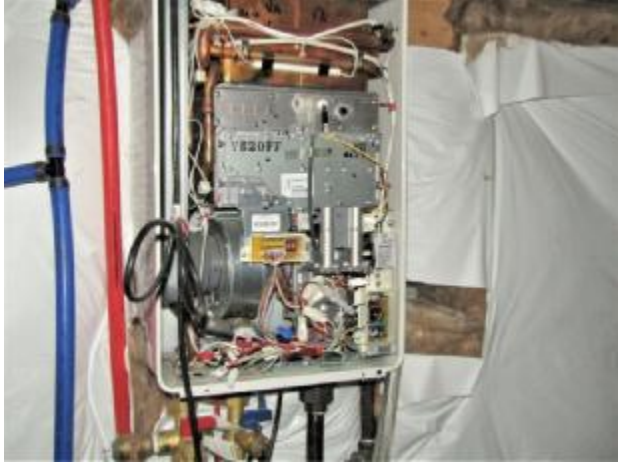
The water heater is working properly but the front cover is not in place.
