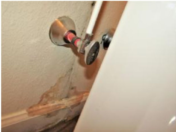
The sink in the downstairs bathroom is loose from the wall and the floor. The sink drain is leaking.
