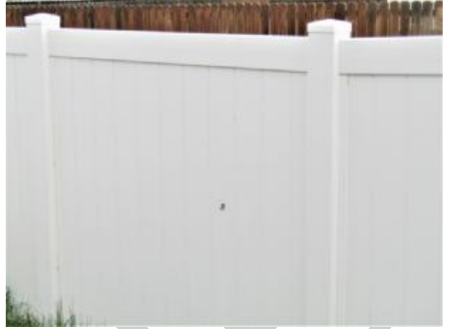
The fence around the backyard has damage.
