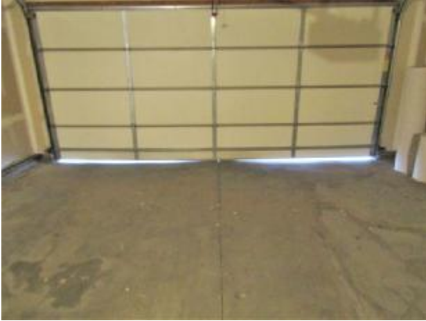
The bottom seal for the garage door is missing. This could cause water and pest infestation.
