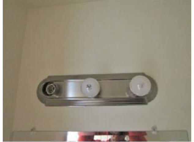
The light in the hallway bathroom is missing a bulb and one is out but the sockets work (need new bulbs).
