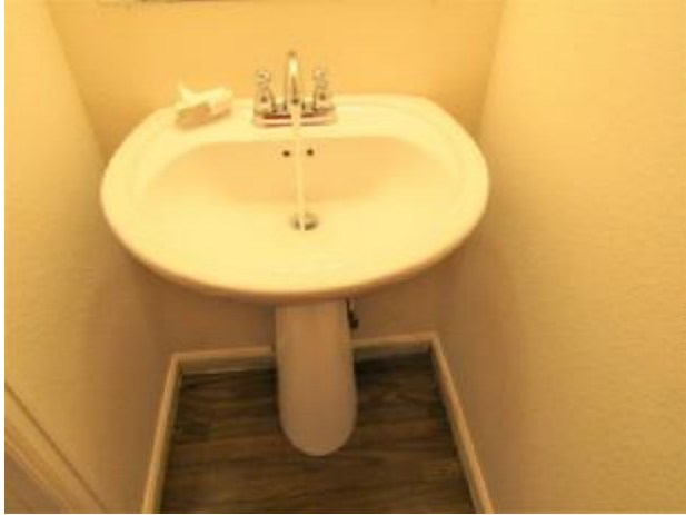
The sink in the downstairs bathroom is loose from the wall and the floor. The sink drain is leaking.
