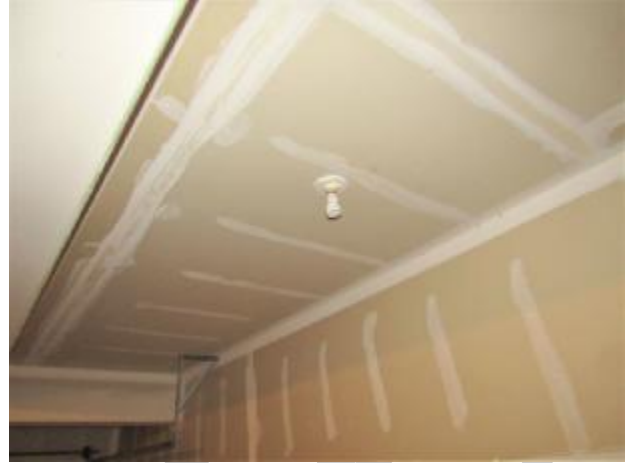
The one ceiling light in the garage does not work.
