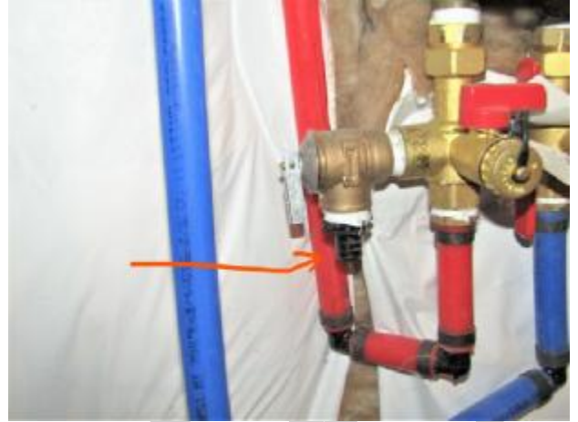
The temperature/pressure relief valve extension pipe is not installed at the water heater for safety.
