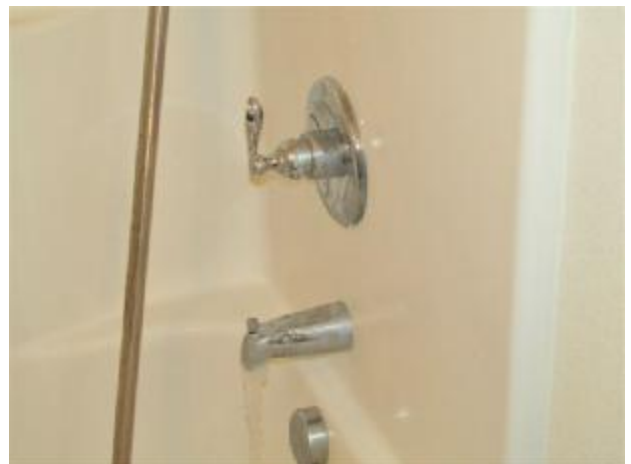
The showers in both of the upstairs bathrooms do not work properly and the faucets need sealed to the wall.
