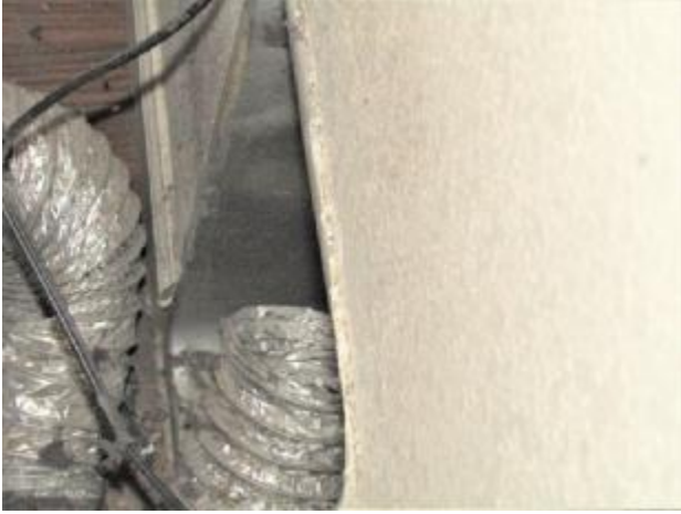
The dryer vent tube is not connected behind the dryer.
